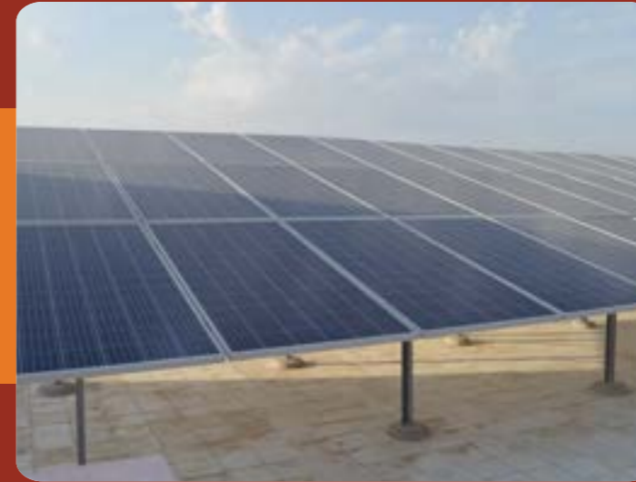
Rooftop Solar Plant
