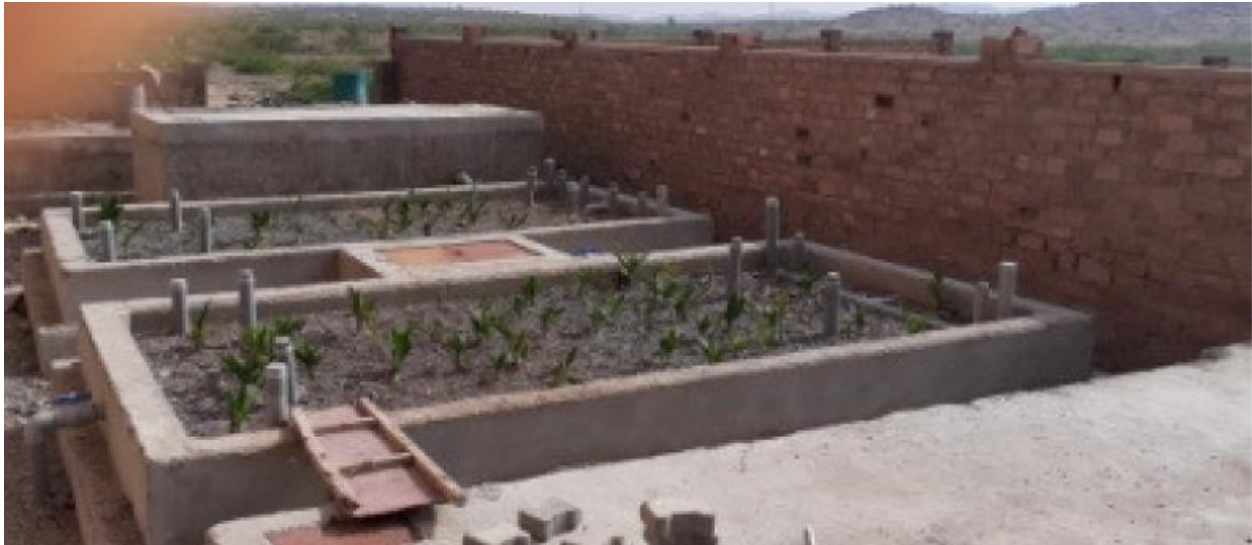
Fig 3: Recently commissioned STP plant
