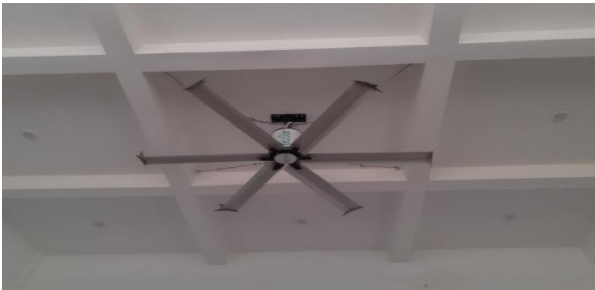
Fig15: Eco Air fan at building reception
