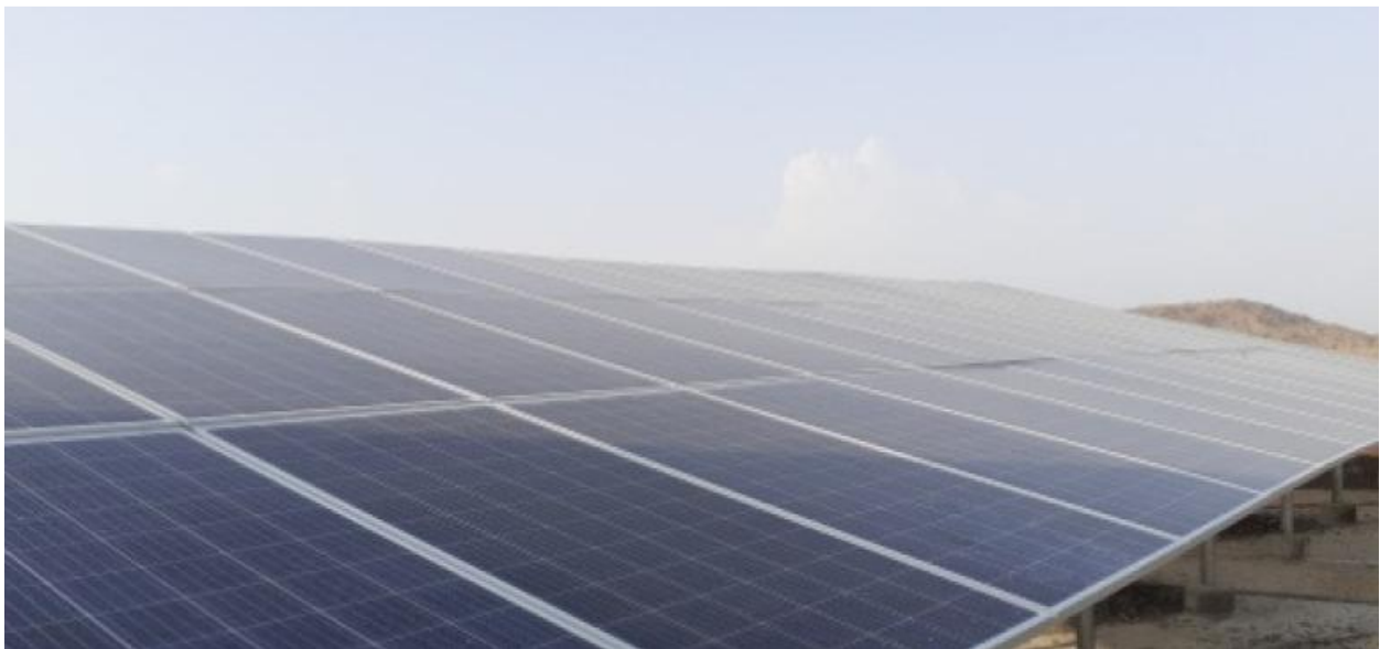
Fig 4: Captive SPV plant 35kWp
